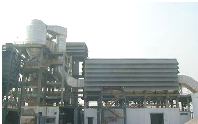
Figure 3. SO 2 Scrubber and Baghouse.
