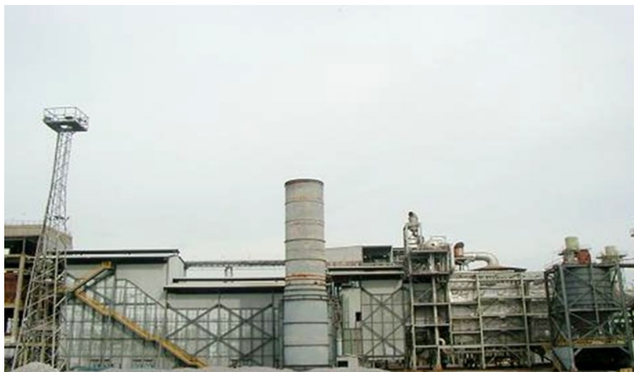
Figure 2. Pyroscrubber and Waste Heat Recovery Boiler.
