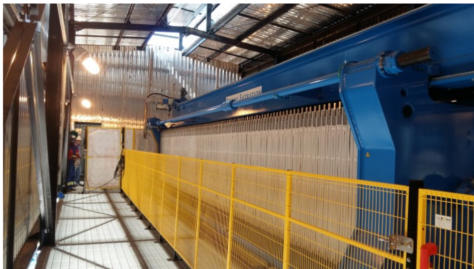
Figure 1. 10 tph Filter Press.
