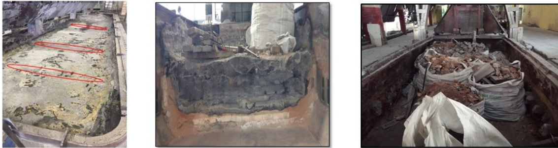
Figure 2. Typical processing steps after pot failure. Left: cavity cleaning after pots failure, Center: layer-by-layer delining for better segregation, Right: segregation of carbon & non-carbon portions of SPL.
