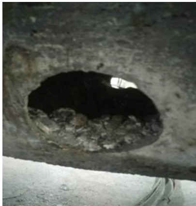
Figure 3. Accumulation of alumina in the duct.
