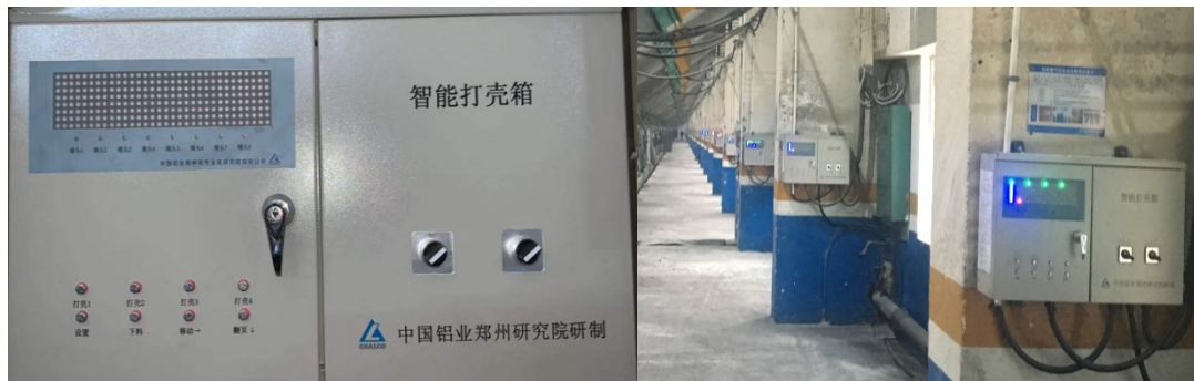
Figure 2. Appearance of intelligent control box and Field installation situation.
