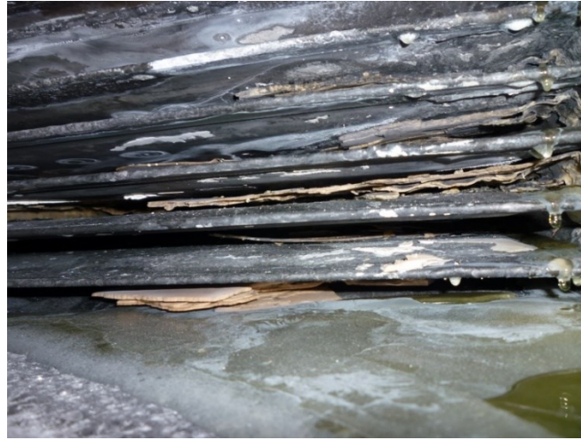
Figure 1. Scale on the heat transfer wall.
