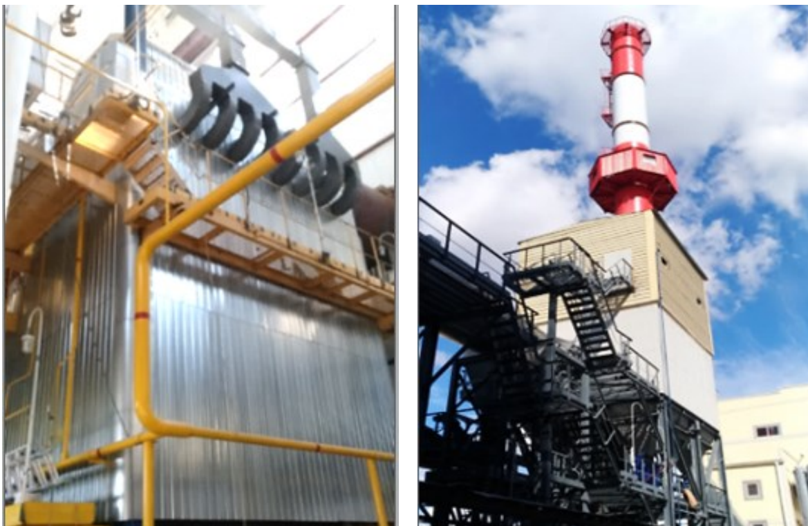
Figure 2. Left: a waste heat boiler, right: a gas treatment centre of the heat recovery facility
