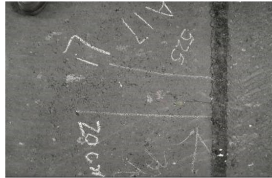
Figure 4. Cracks in Pot #1534 B18.
