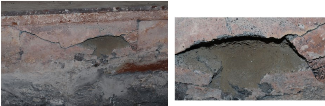
Figure 2. Example of severe degradation due to bad quality sidelining material. Plant B.
