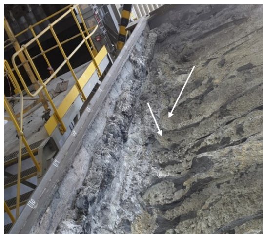
Figure 7. Erosion pattern and indication of vortices.
