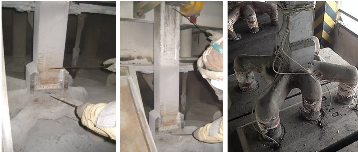
Figure 12. Monitoring of the voltage drop in the 'rod–yoke' contact of bimetallic plates mounted according to type 5.
