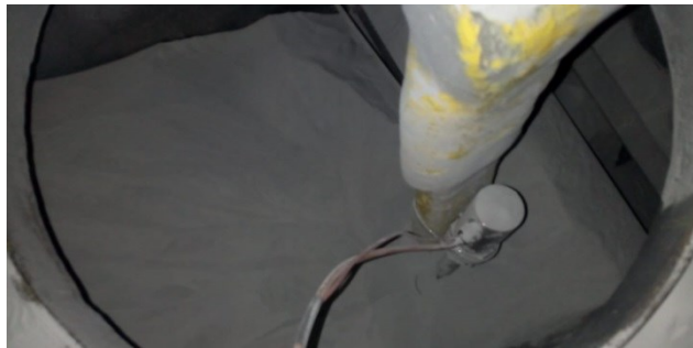
Figure 12. High-level sensor used to stop the air compressed when pot's last silo was full.
