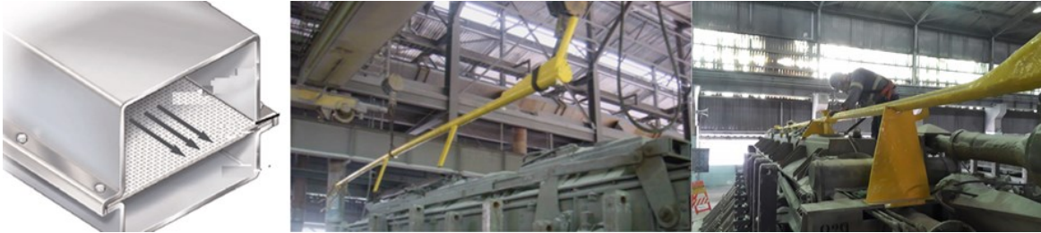
Figure 7. The Albras aluminum smelter air fluidized conveyor (center and right) and a conventional air slide (left) [6].
