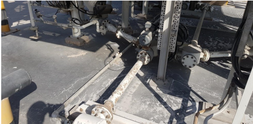
Figure 12. Hammer marks on a dense phase system.
