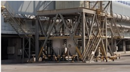
Figure 5. EGA Jebel Ali Potline 9 dense phase system.
