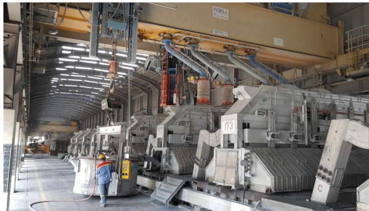
Figure 4. EGA Jebel Ali Potline 5 with simultaneous alumina fill and metal tapping.
