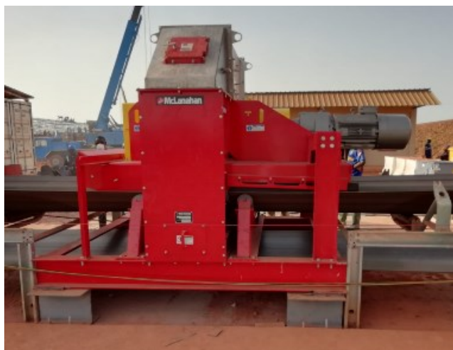
Figure 6. Automating Sampling system during ship loading was installed.
