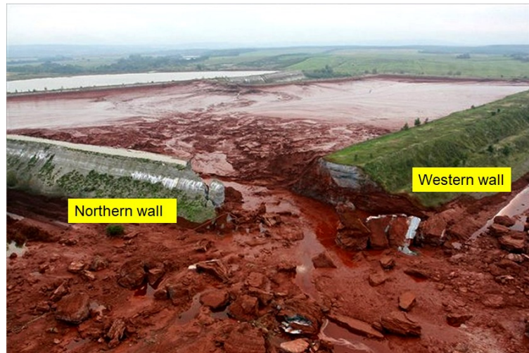
Figure 2. General view of Reservoir 10 one day after the failure of the embankment.
