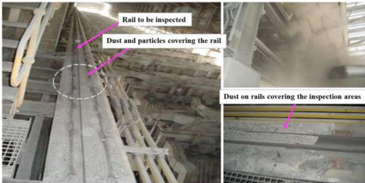
Figure 2. Building rail and associated hazards (dust and fumes).
