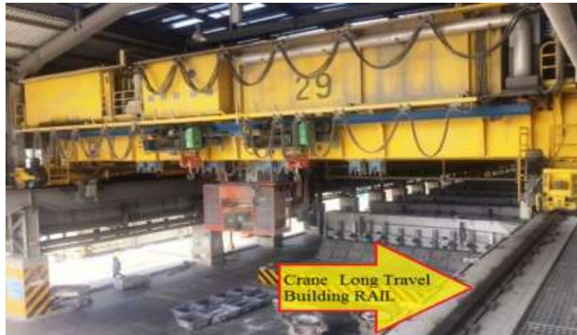
Figure 1. One of the potroom cranes in operation, the picture shows building rail.
