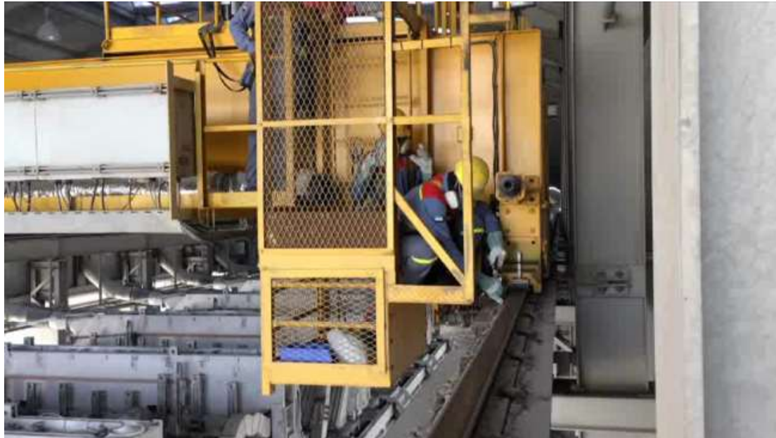
Figure 9. Picture shows maintenance crew using pneumatic torque wrench for tightening and replacement of rail clamps.
