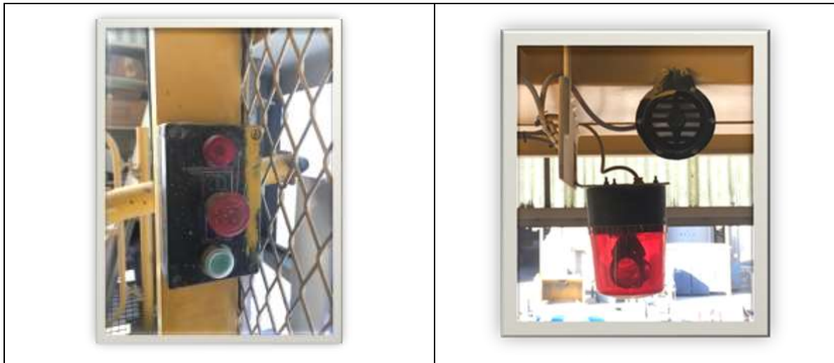
Figure 7. Left: safety stop and horn, Right: visual and audio alarm.
