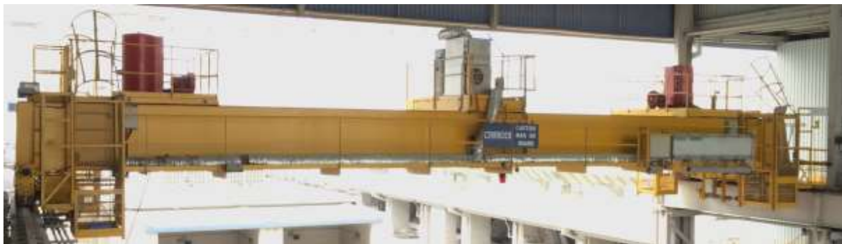
Figure 4. Building rail inspection car parked in crane maintenance bay.
