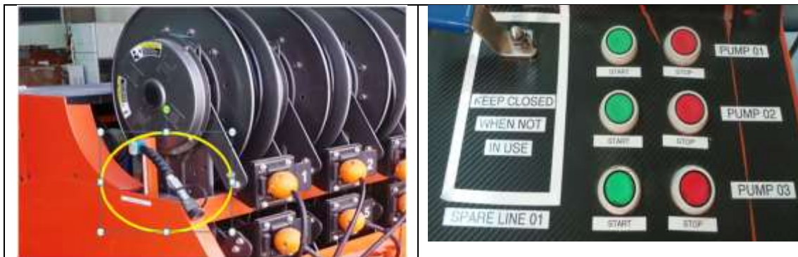
Figure 11. Left: emergency hose line, right: push buttons.
