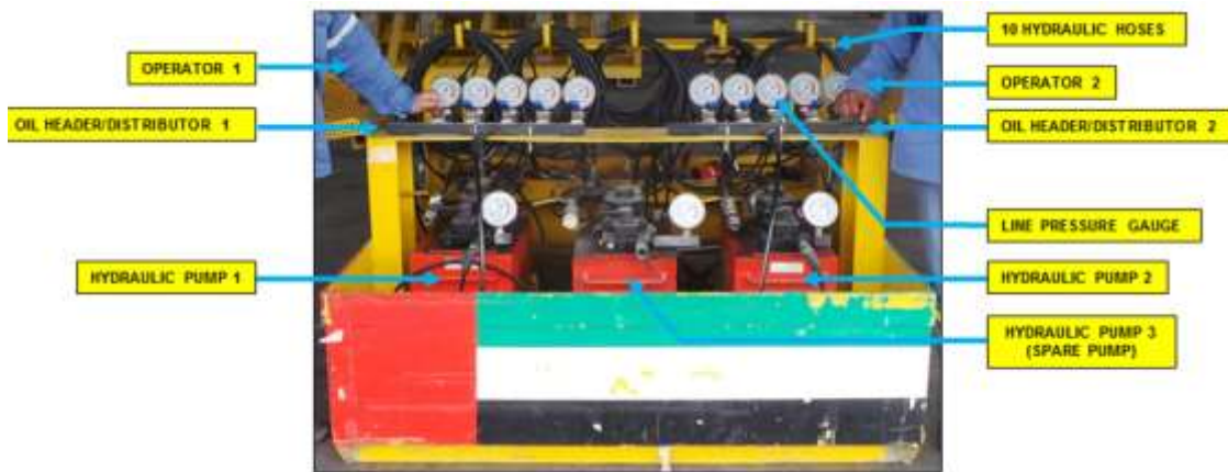
Figure 3. Original wedge puller hydraulic unit in EGA AT Potline 3.
