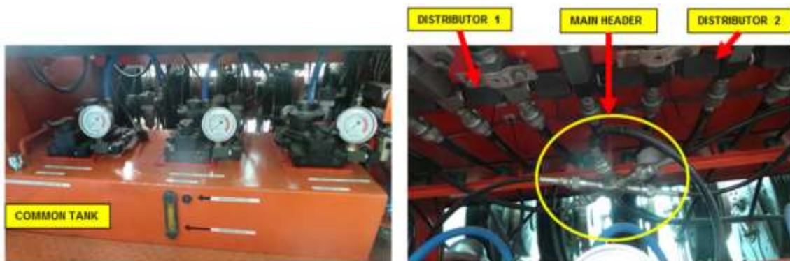
Figure 8. Three individual hydraulic pumps (left) with common outlet header (right).
