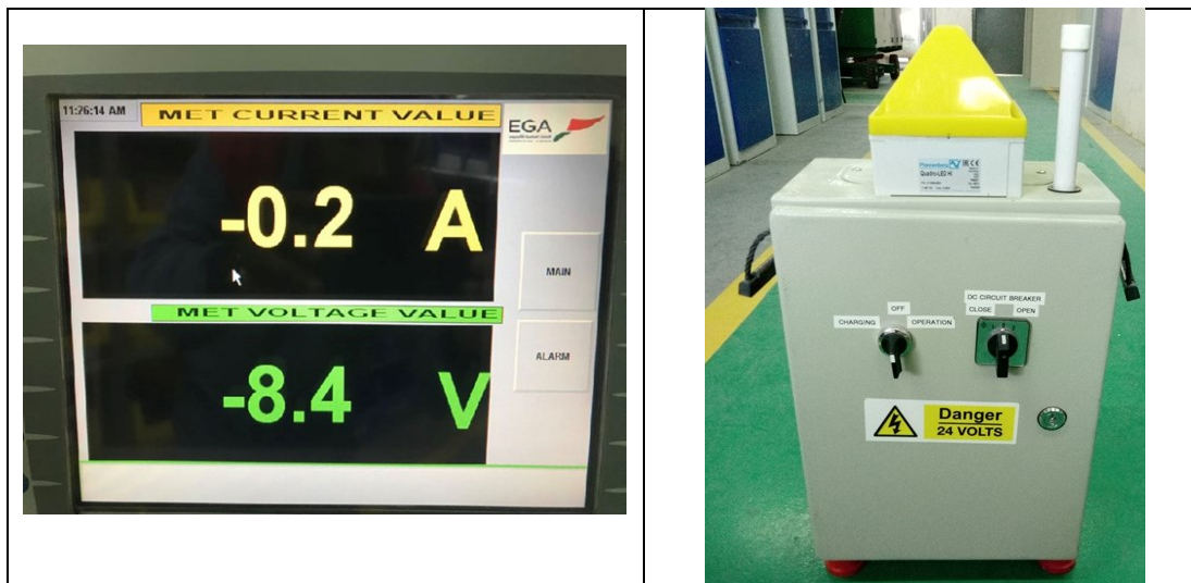
Figure 7. SET voltage and current display (left) and wireless flasher module (right).
