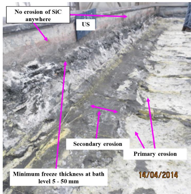
Figure 10. Sidewall of Al Taweelah Pot 2B002 autopsy, showing elements of good thermal equilibrium during lifetime.
