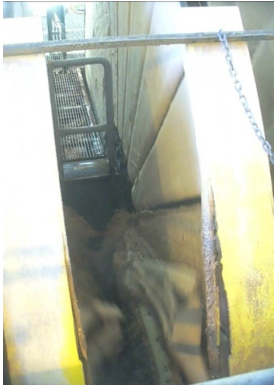
Figure 6. Spoke wheel with polymer segments in operation (cake discharge)
