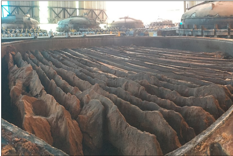
Figure 1. Scale on top of the pressure leaf filter before filter bag refurbishing.
