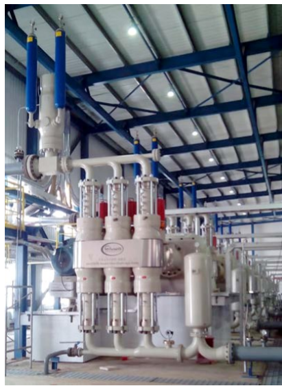
Figure 1. Seven sets of double hose-diaphragm pumps.
