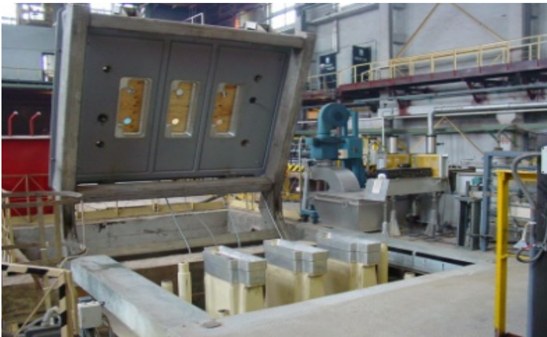
Figure 3. Underside of Hatch Hot Top mould table free from water hoses.
