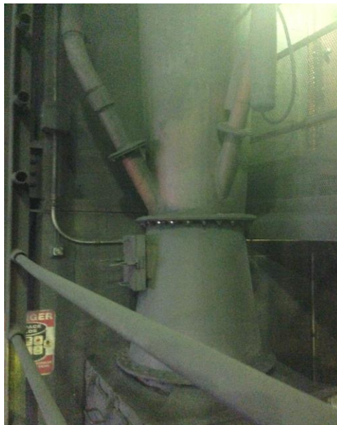
Figure 1. Fresh and loaded coke injection points at venturi throat before dust collector
