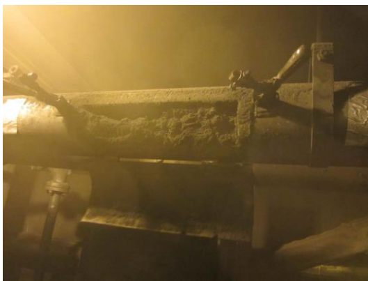
Figure 4. Ventilation duct before fine coke injection point implementation
