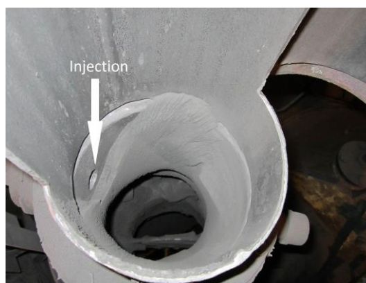
Figure 3. Duct with injection point, showing accumulation
