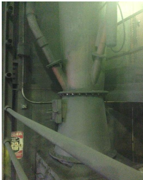
Figure 1. Fresh and loaded coke injection points at venturi throat before dust collector
