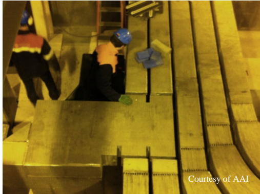
Figure 22. Interlinked connections used in Iceland.
