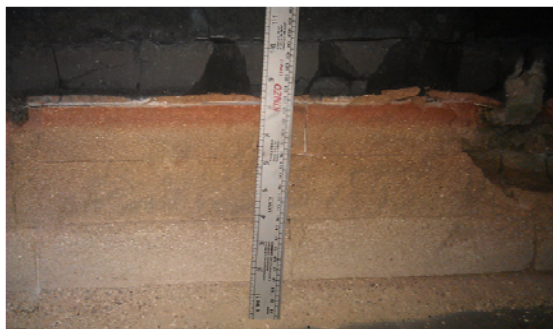
Figure 4. Condition of Insulation and Refractory Bricks, Cathode of Cell A.
