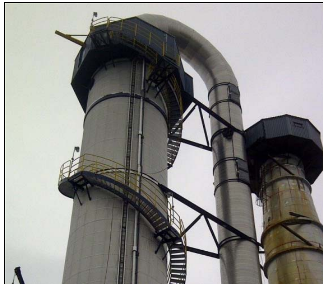
Figure 9. New conditioning tower alongside existing tower.
