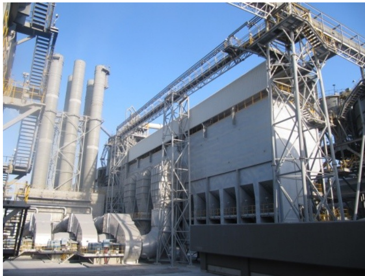
Figure 12. Centralized GTC with seawater desulphurization (SWFGD) scrubber.
