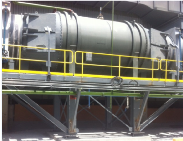
Figure 4. Heat exchanger for pot gas cooling.
