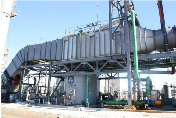
Figure 2. IDS system at Lake Charles.
