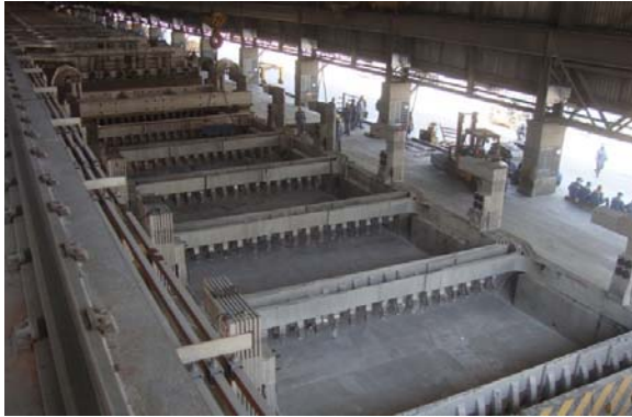
Figure 7. Original busbar after removal of D18 Technology cells.
