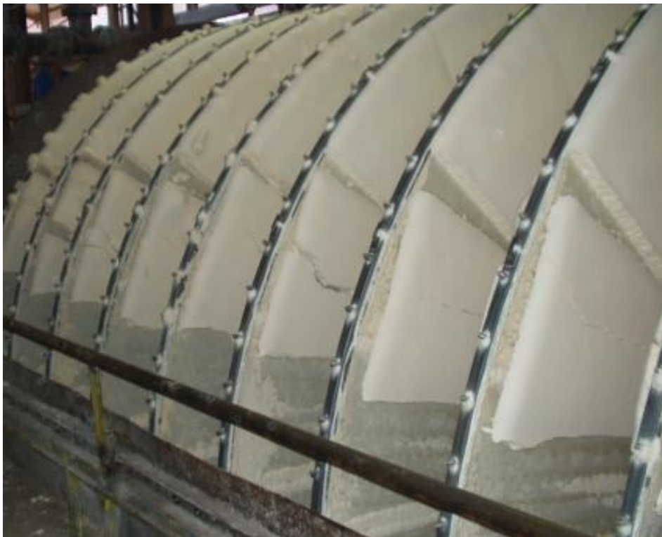
Figure 6. Complete cake discharge of a type A disc filter after revamping with “large package” modifications
