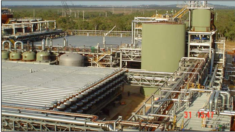
Figure 4: Yarwun Stage 1 Tube Digestion Facility - 2004
